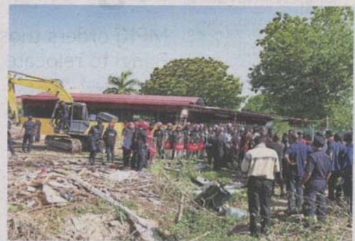
FRU personnel on standby at the site of the Hindu shrine which was demolished in Bandar Botanic Klang.
